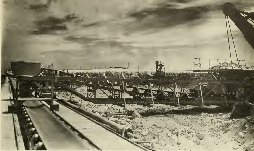
Belt Conveyor at Vat Site.
